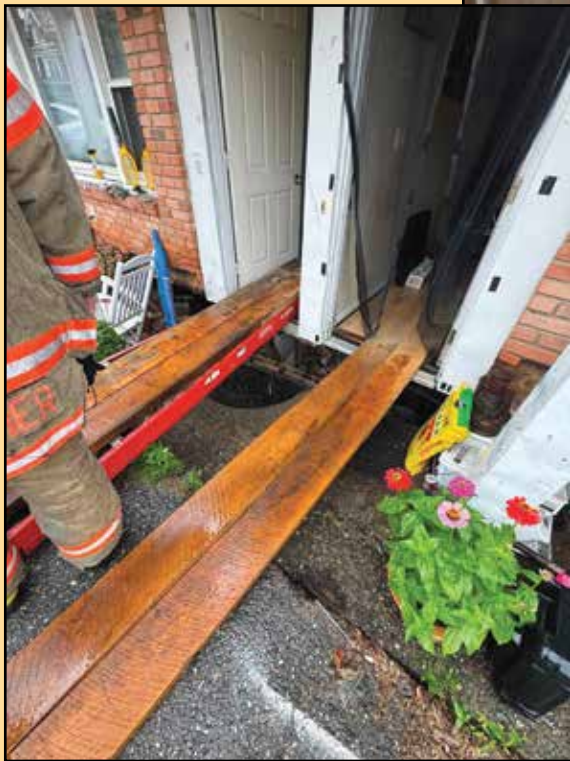
A multi-family building on See Avenue in Mahopac partially collapsed July 6 due to water damage, leaving three families temporarily homeless. Crews used planks to help residents safely exit the building.
