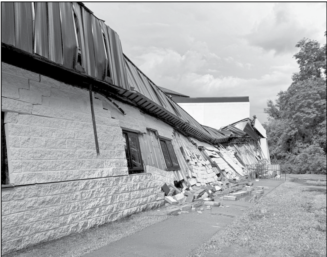
The Hudson Valley InterArts building at 40 Jon Barrett Road in Patterson was damaged in last week’s torrential rain. Photo by Patterson Fire Department.
