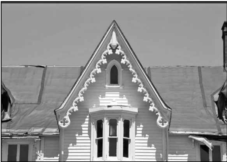
The Belden House has been in disrepair for years.
